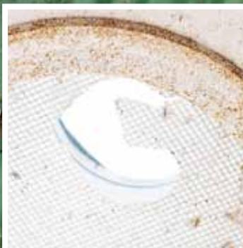
One of John's plastic dome skylights from the inside: hail stones crashed right through.
